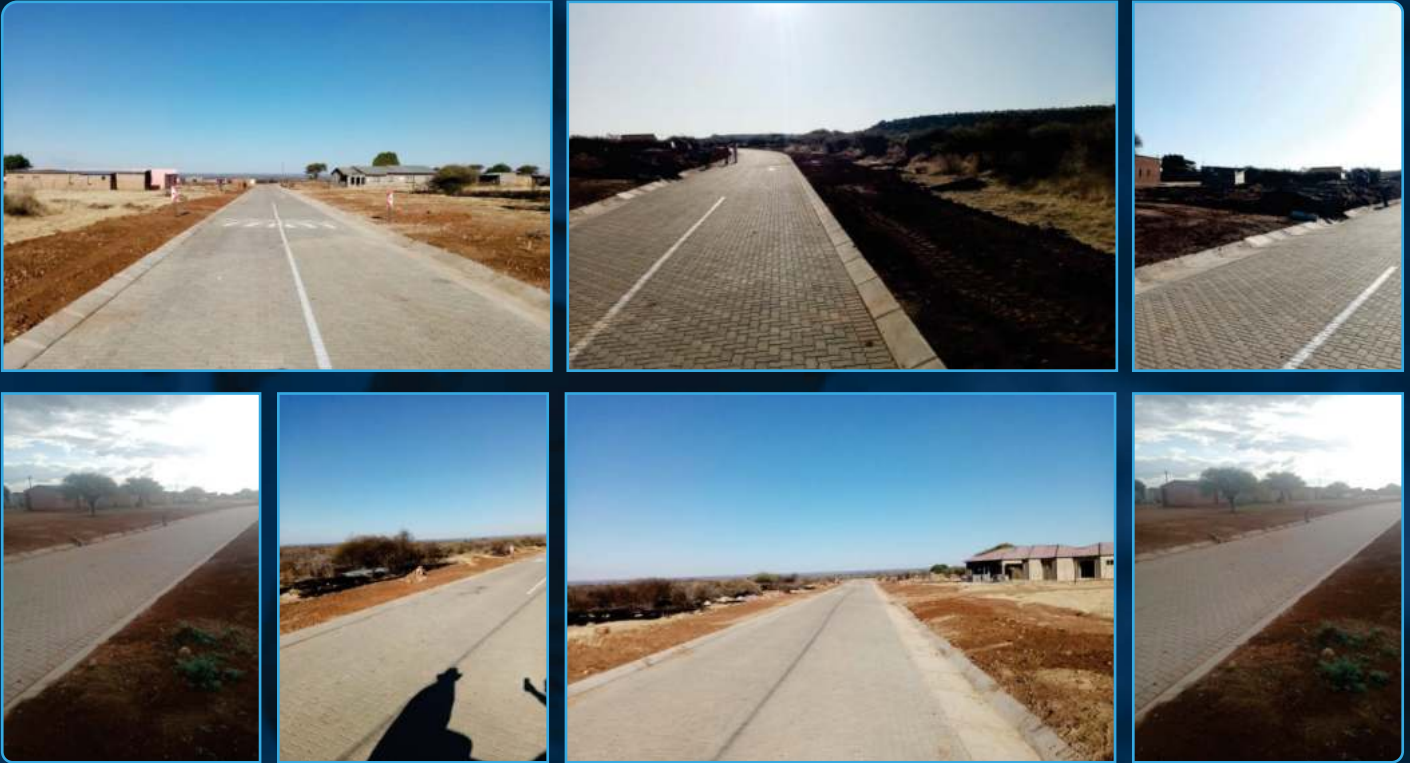
Client - Greater Taung Local Municipality Project - Construction of Upper Majeakgoro Access Road Year - 2022
