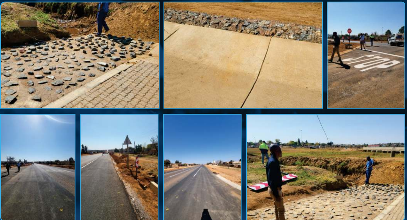
Client - Thembisile Hani Local Municipality Project - Construction of Mandela Luthuli Bridge Road -Ward 22 Year - 2022
